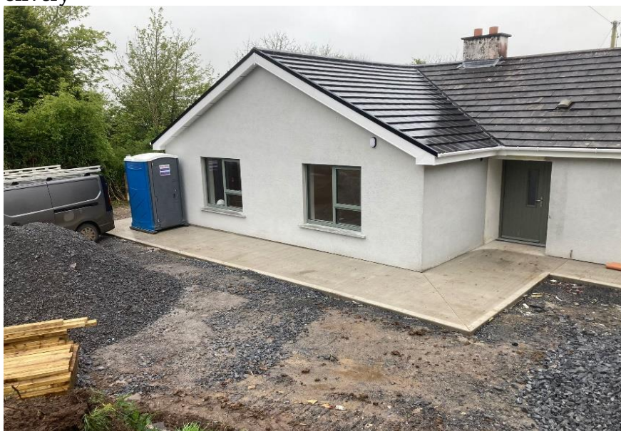
Adaptation of an existing bungalow at Closhgregg, Thomastown to a Disability Unit
