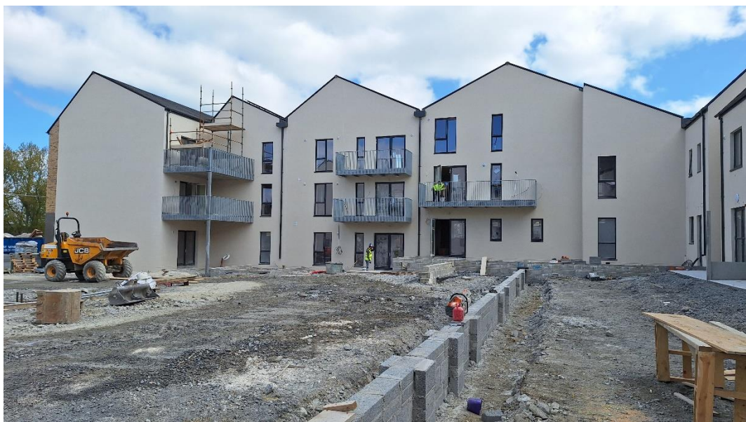
Construction ongoing at Crokers Hill, Kennyswell Road. Due for completion this year.
