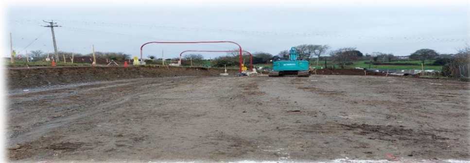
Site Works at Ladywell Thomastown - John Somers Construction - 25 units for Kilkenny County Council
