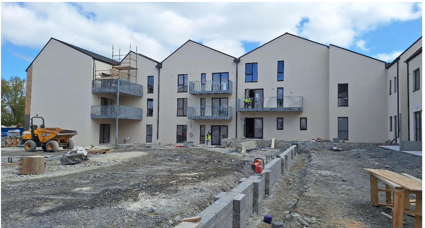
Construction ongoing at Crokers Hill, Kennyswell Road. Due for completion this year.
