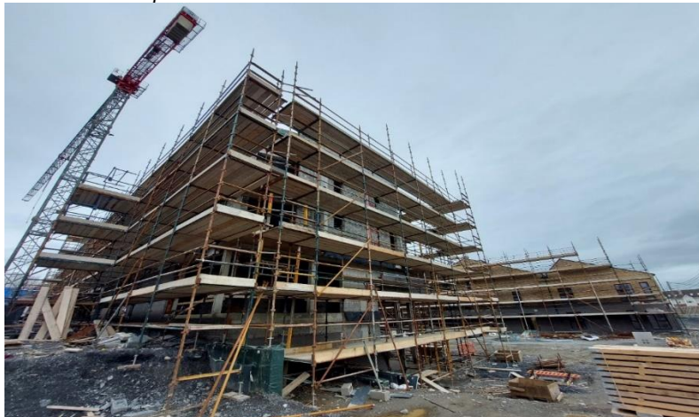
Construction ongoing at Crokers Hill, Kennyswell Road. Due for completion this year.
