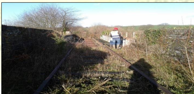
Examining one of the old bridge structures along the route of the South East Greenway at Carrickcloney
