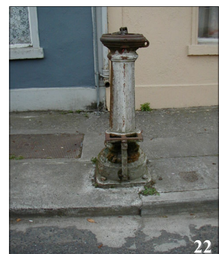
Photo 22: Disused water pump on New Line Street.
