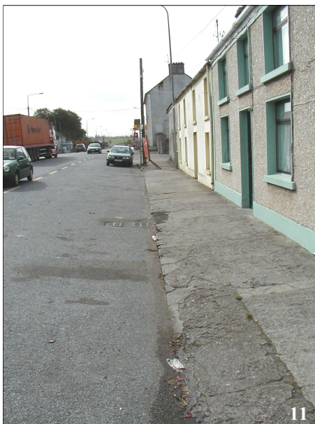
Photo 11: Example of poor footpath conditions on the north side of Main Street. Note width of road margin - significant opportunities exist for widening the pavement, with designated parking bays and street trees.
