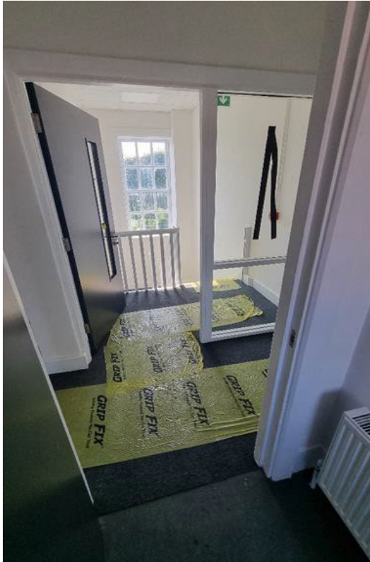
Fig.31 – Fire door and screen to stair enclosure
