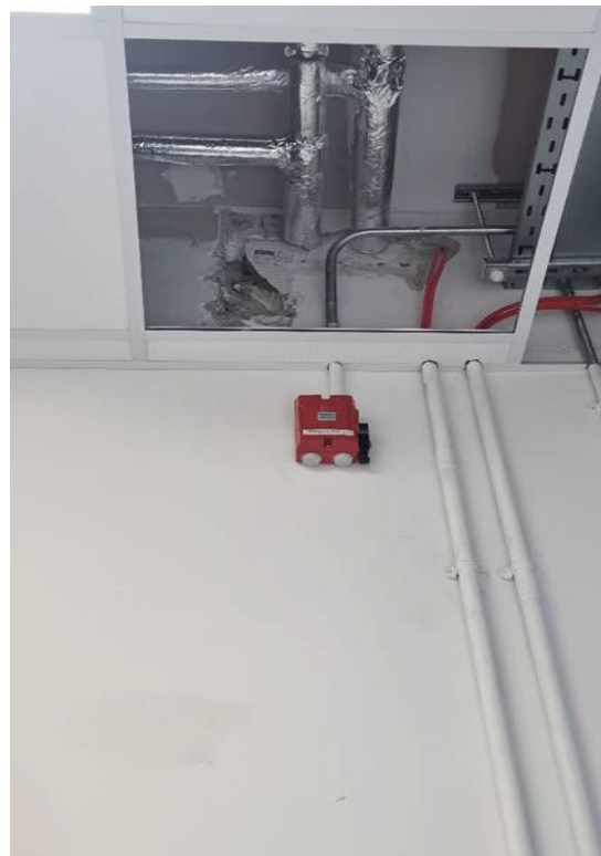
Fig 34. Fire stopping to escape routes
