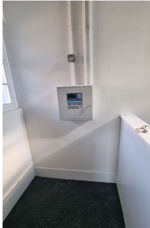
Fig.32 - Fire alarm panel
