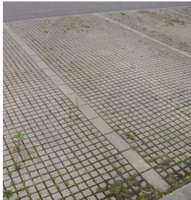
SUDS - permeable parking areas
