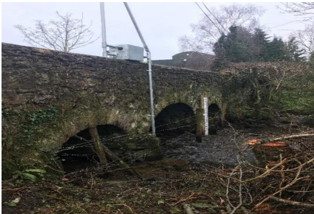
New Water Level Gauge – Coolroe
